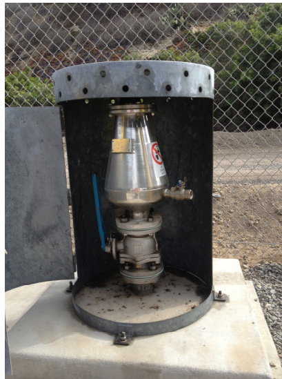
FIGURE 12. 3-inch intermediate air valve (Courtesy of OCSD).
