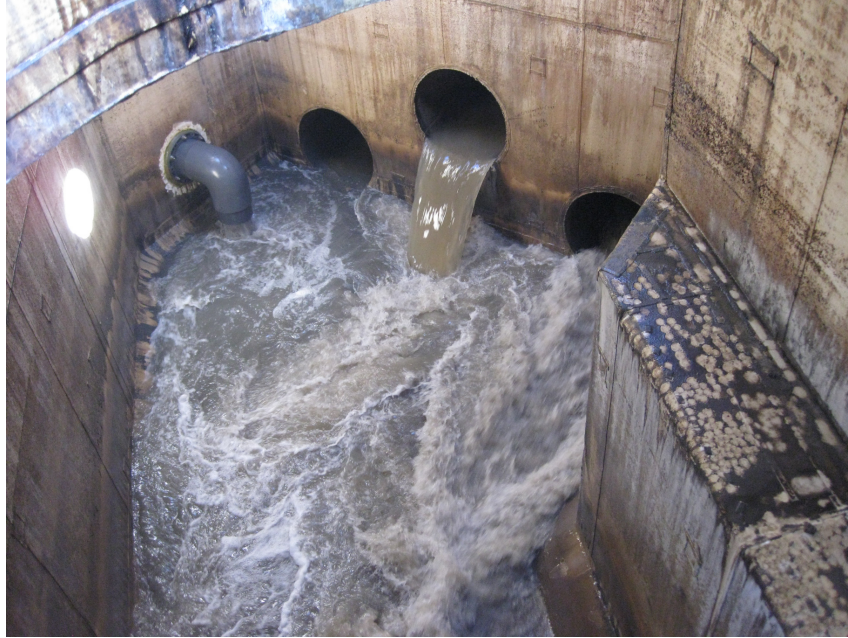
FIGURE 5. Plunging jet into wet well (Courtesy of OCSD).
