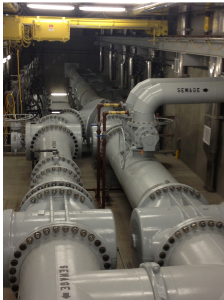
FIGURE 10. East and west force mains (Courtesy of OCSD).
