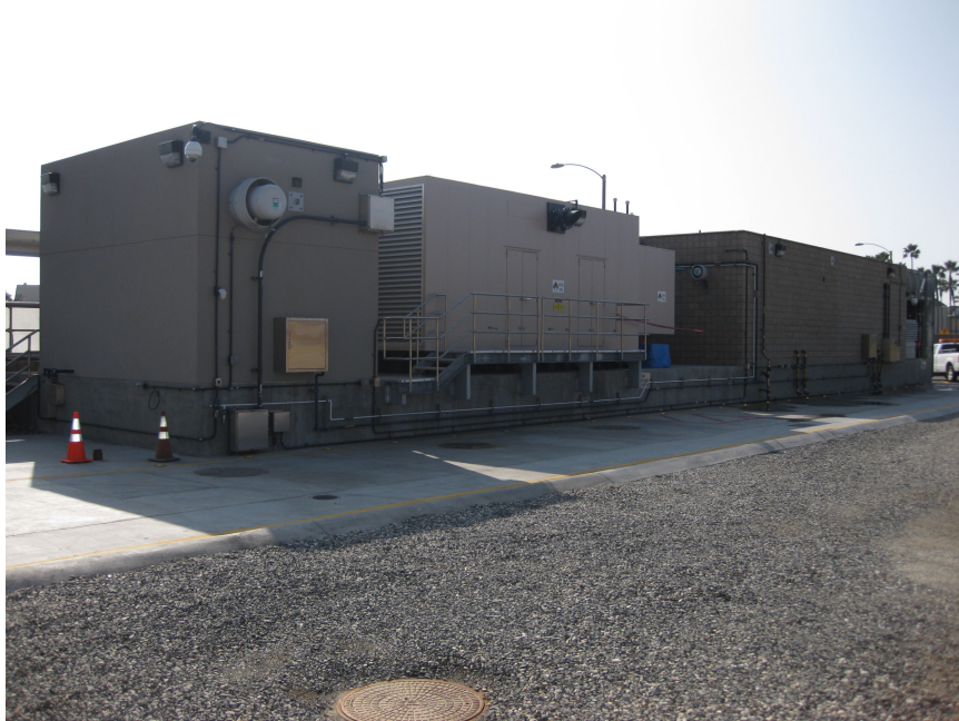
FIGURE 9. Bitter Point Pump Station in Newport Beach (Courtesy of OCSD).
