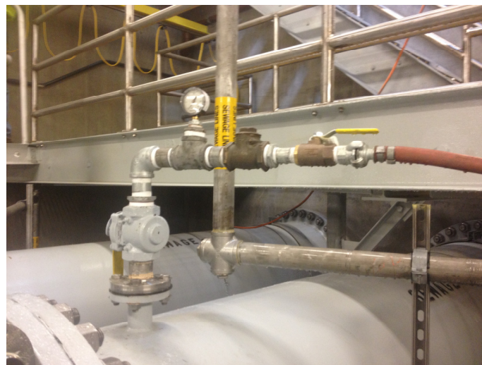
FIGURE 15. Air injection port (Courtesy of OCSD).
