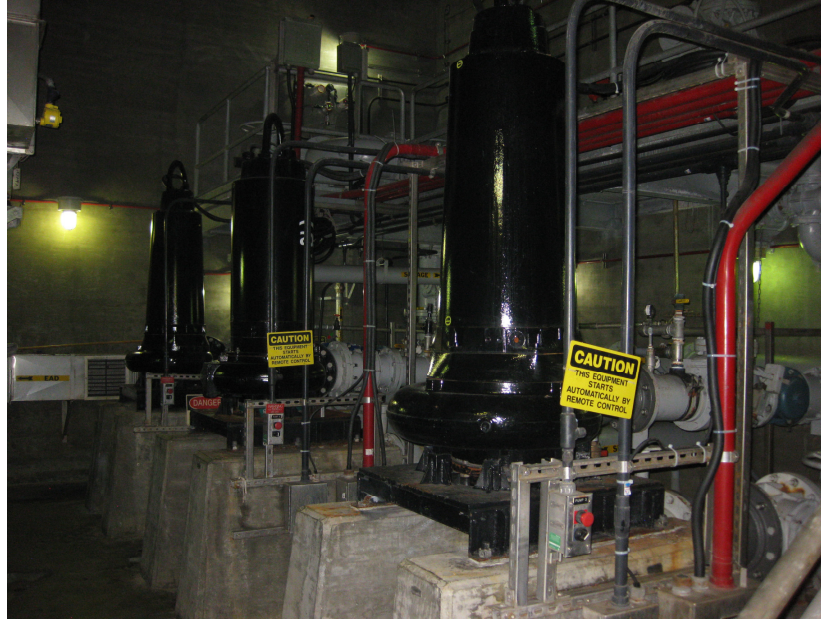
FIGURE 8. Lido Pump Station pumps (Courtesy of OCSD).
