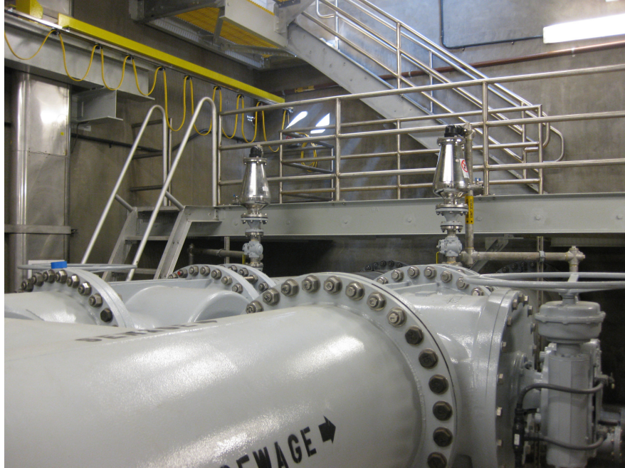
FIGURE 11. 4-inch air valves on east and west force mains (Courtesy of OCSD).
