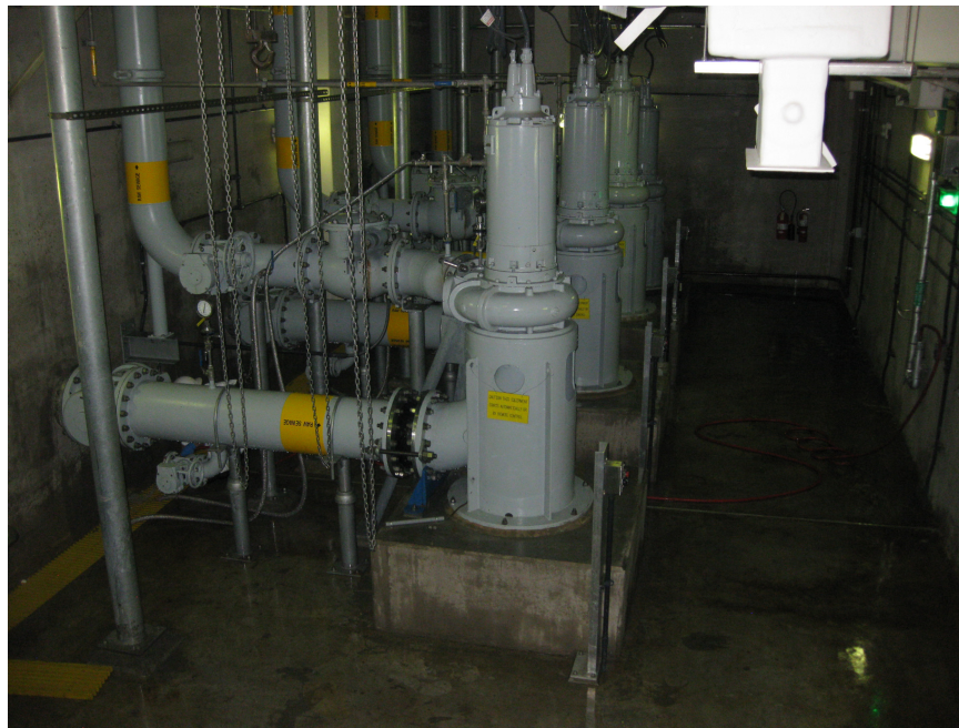
FIGURE 7. Rocky Point Pump Station pumps with suction and discharge piping (Courtesy of OCSD).
