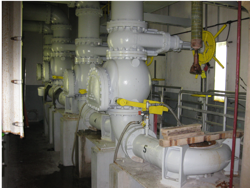
FIGURE 6. Bay Bridge Pump Station valves and discharge piping (Courtesy of OCSD).
